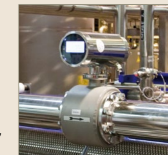
Metering technology for the filler lines
